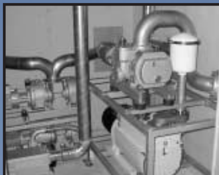
Compact Oil Mist Exhaust Filter Mounted on a Vacuum Pump
